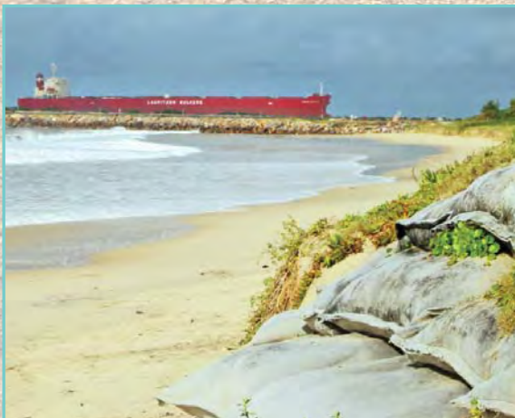
Exposed ELCOROCK ® containers post June 2007 storm event
